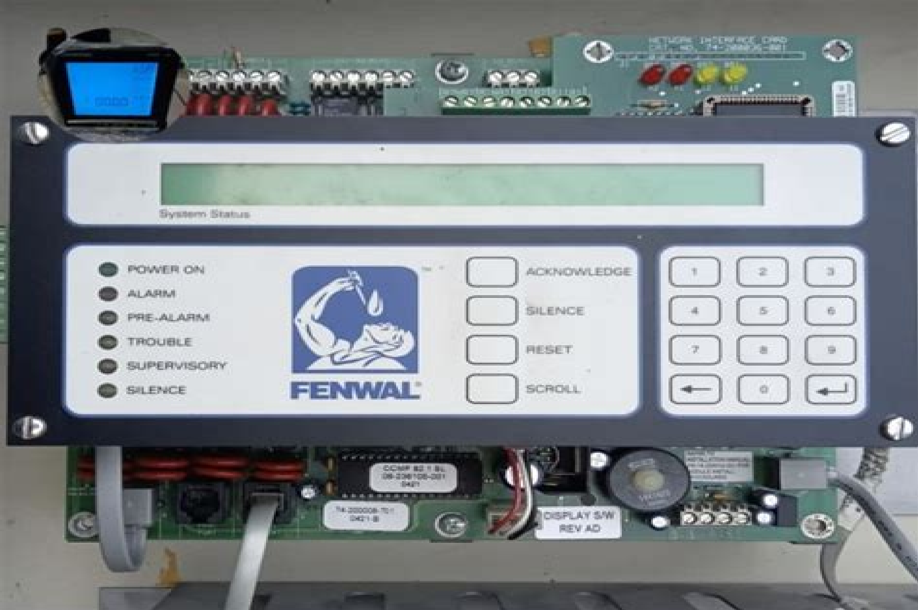
Fenwal Main Control Panel 74-200008...
