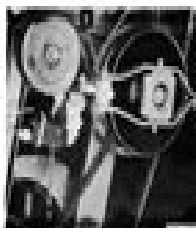
Fan protection (Shield removed)
